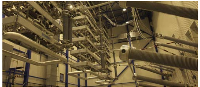
Püssi converter station valve hall
